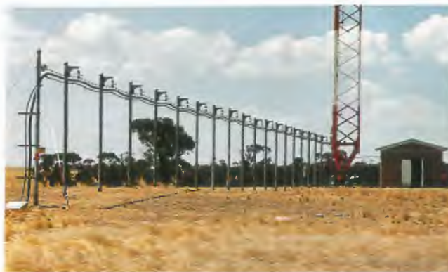
The 140 metre long elevated short circuited quarter wave stub.
