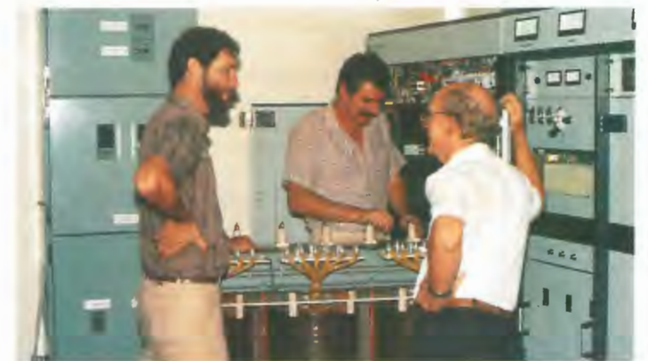
BRISBANE L to R, Des Eckford OIC Installation, Dave Boreham, Chris Jeffrey OIC ABQ2.
