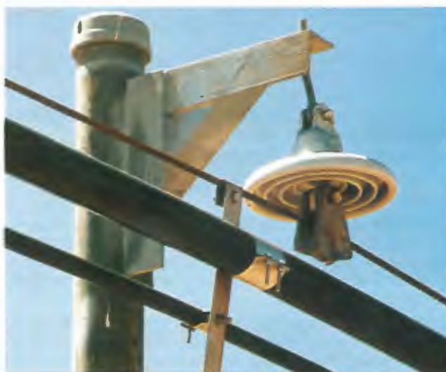
Details of support for insulated catenary wire carrying live coaxial cables.
