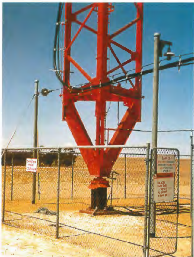
Base of 6DL mast showing transition of TV cables from the insulated catenary wire to the live mast.
