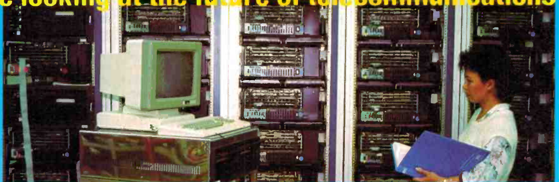
Testing a complete X25 Package Switching Exchange
