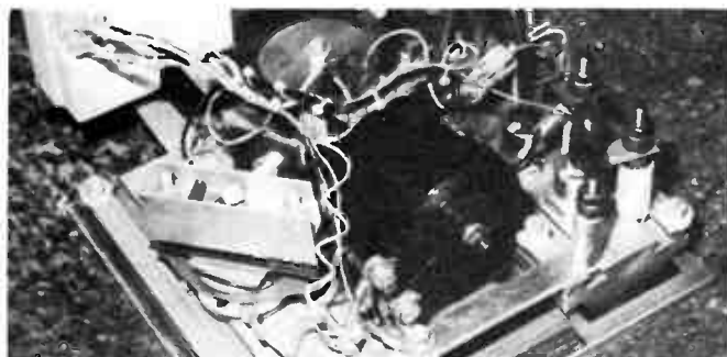
Semi-conductor controller for a dc motor system. (Photo: NSW Dept of Energy.)
