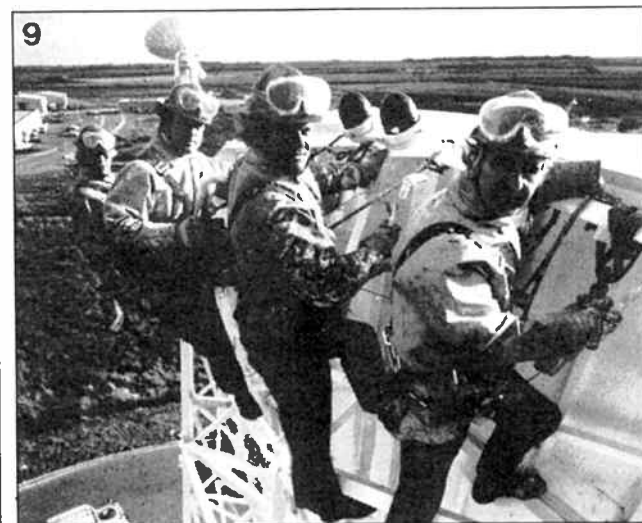
Fig. 9. The antennas are painted regularly: each one takes a 1000 gallons of marine paint and two full seasons' painting. Photograph courtesy of British Telecom.
