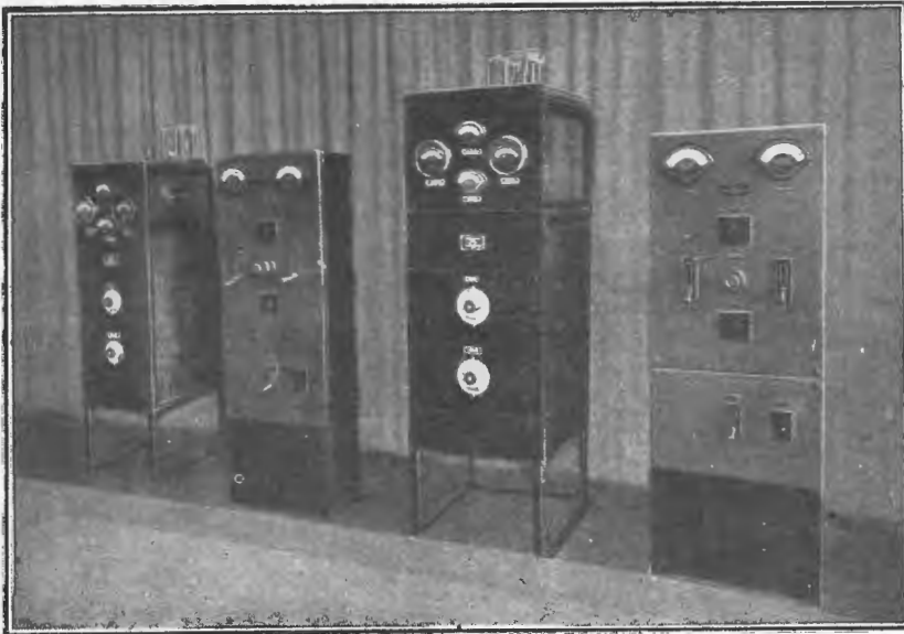
BROADCASTING EQUIPMENT AT THE NORTHERN ELECTRIC CO'S. BROADCASTING STATION IN MONTREAL.
