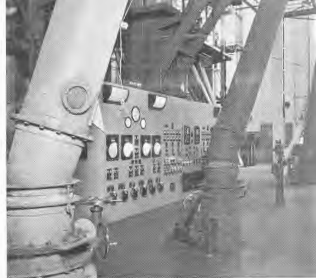
The automatic-electric-pneumatically controlled raising plant.
