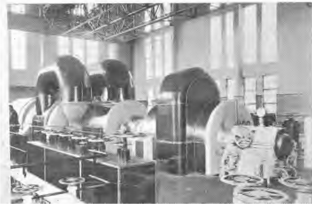
Another view of the generating equipment.
