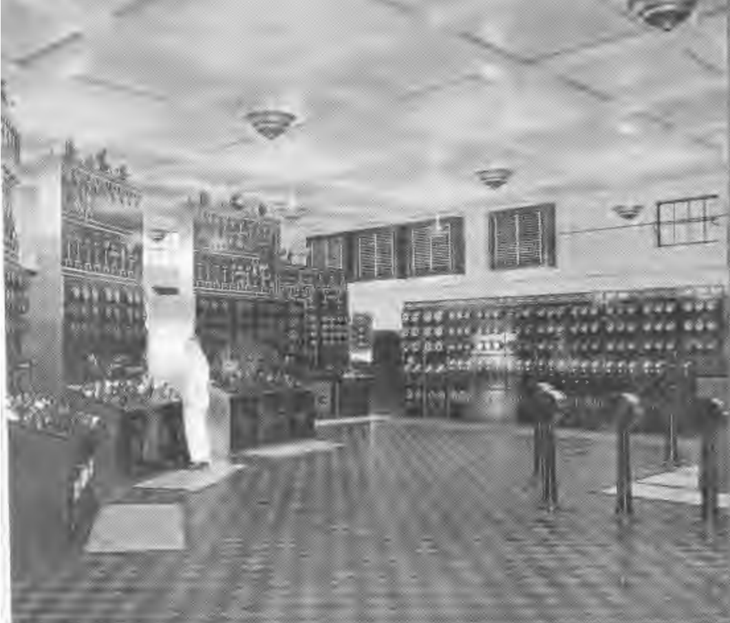
The main control room, Bunnerong Power House.
