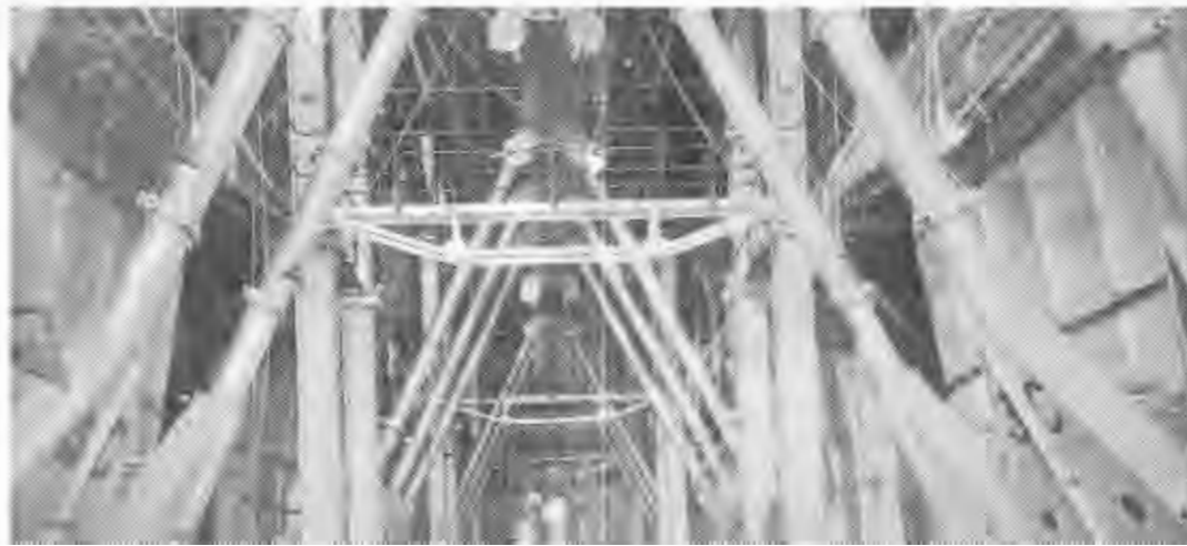
The boiler firing aisle. Furnaces are ignited by a 10,000 volt sparking device.
