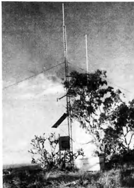
VK4 Repeater Highland Radio Finished. There is a pole on top of the tower to act as a lightning arrester, 70 centimetre antenna, two metre link folded dipole, solar panel, repeater housing and an old refrigerator for the battery.
