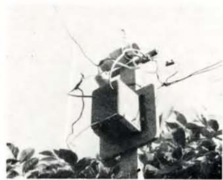
Loop tuning box and coil, 12 ft. from ground.
