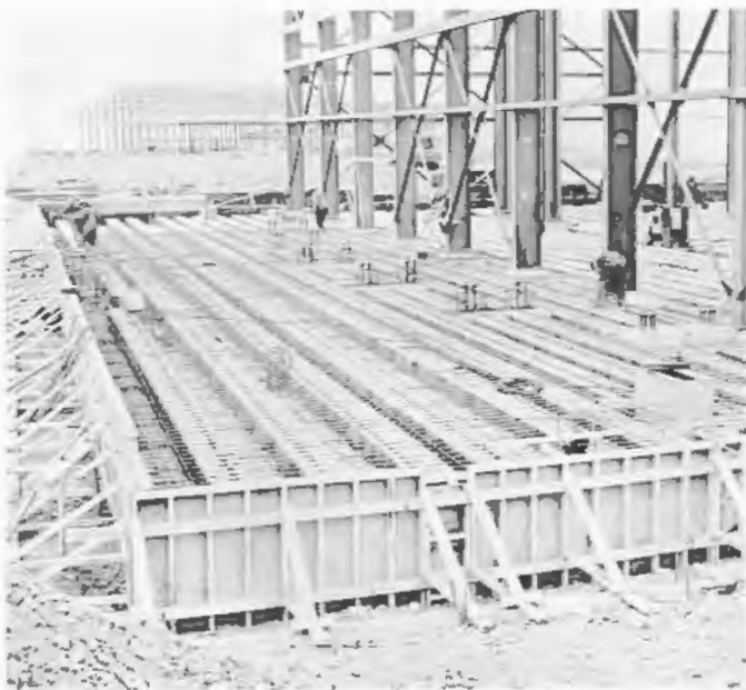
Greenland Site #1—Buildings 5 and 1 (in background) are constructed of structural steel to withstand the area's 135-mile gales.
