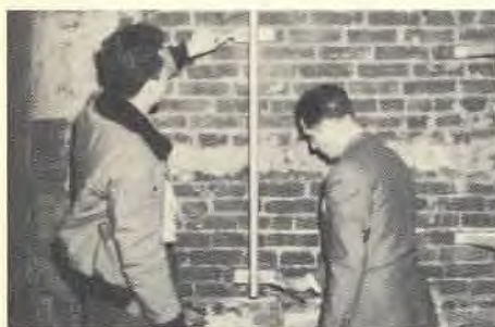
Trainees J. P. Lozascio and W. Finkbeiner work on installation using pipe straps.
