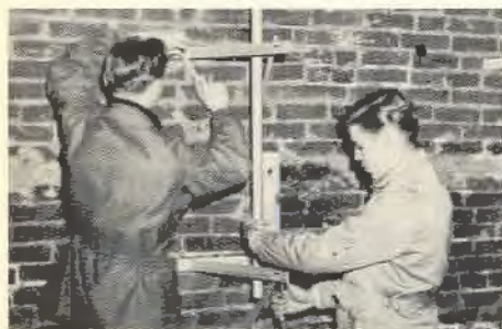
Trainees R. Kaltenbough and L. R. Lindsey work on installation using #227 brackets.
