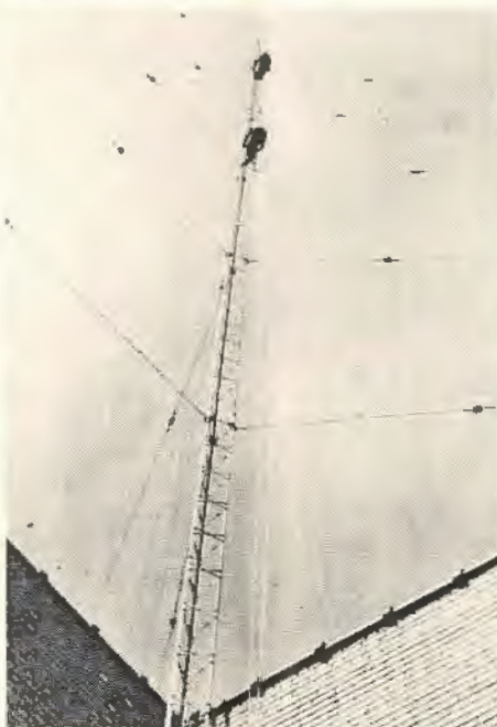
The above photo shows John Dickey at top and Fred Coble completing installation of the antenna.
