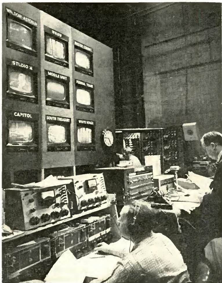
Fig. 4—The switching center in the Wardman Park Hotel. The producer's position is at the right.
