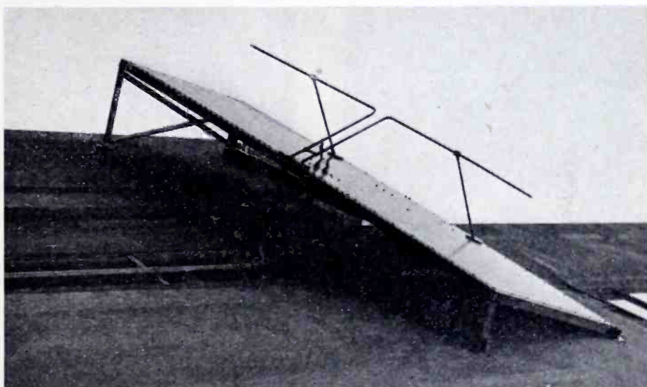
Fig. 2—Transmitting antenna at 14th floor level of RCA Building.
