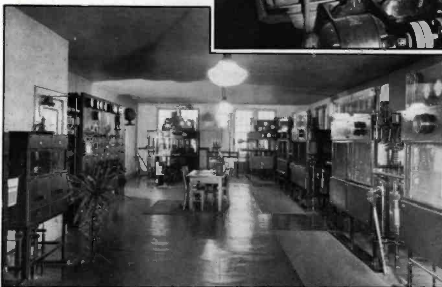
Transmitter of WJZ showing radio frequency equipment, modulators and rectifiers. The large panel on the left controls the incoming power and component parts of the transmitter.
