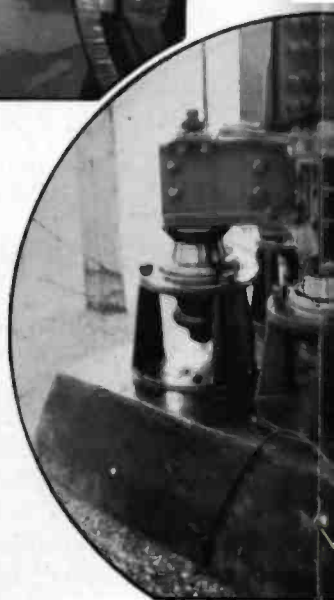
Insulated tower footings which are used at WJZ. Four of these footings are used on each tower to prevent ground currents from affecting the field pattern by the tower.
