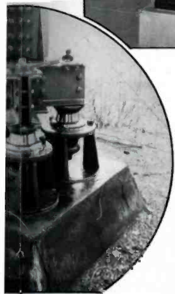
which support the antenna system these footings are employed for prevent distortion of the n by tower radiation.
