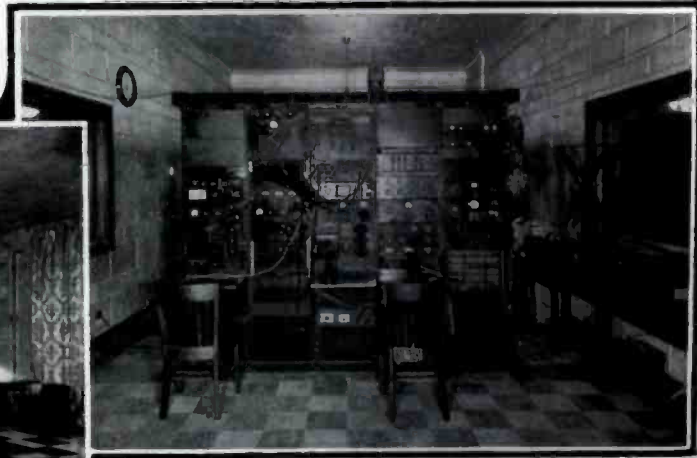
Above: Showing the enormous stage switchboard in the new Atlantic City Auditorium
