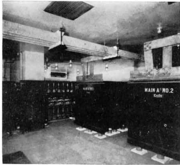
Figure 33. Fifty tons of storage batteries, "A" and "B," which are operated float-charge with the motor-generator sets in the power room.
