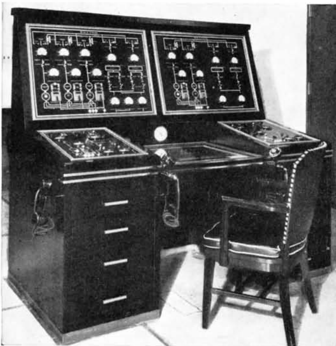
Figure 32. The power control desk showing the miniature supervisory equipment on the panels.
