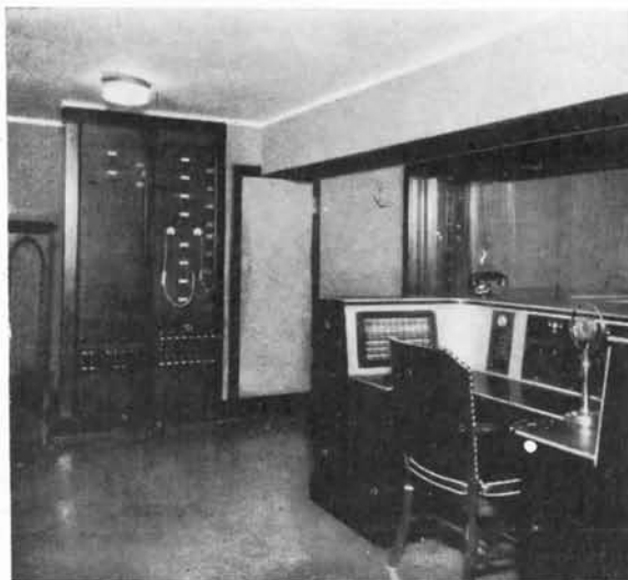
Figure 34. A studio control room showing the loudspeaker, amplifier racks, and the control console.
