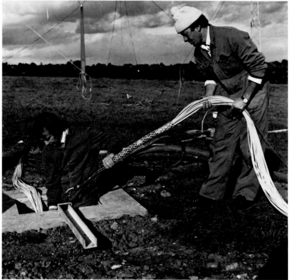
Fig. 6. Installation of the cable ducts. This shows the cable sock that attaches the draw rope to the cable bundle.
