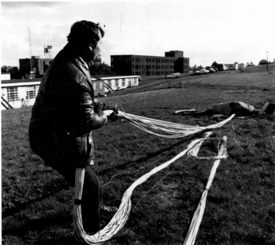
Cable pulling. The cable bundle is pulled through the duct and is guided over sharp edges to prevent damage to the fibers.
