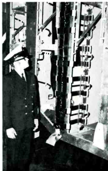
Fig. 19—Emplacement of the analog cables on the rear flange of one column. The assembly shown is repeated on each of the four main vertical flanges.
