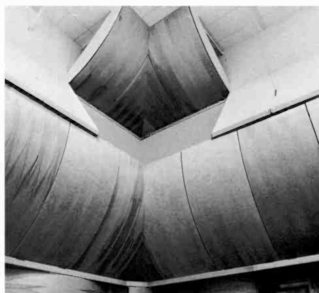
Fig. 15—Closeup view of one of the ceiling corners.
