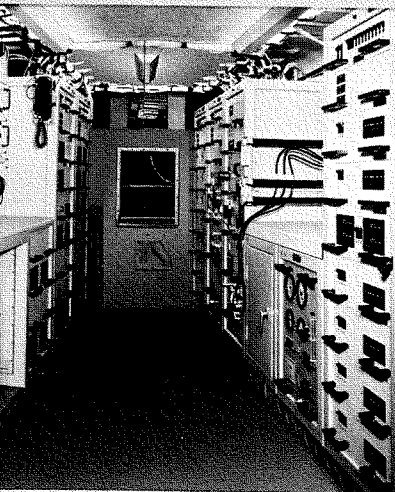
Fig. 2—ETS-2 is used for testing microwave units. The unit is placed on the work surface of the operator control console (shown at the left) and is connected to the test set.
