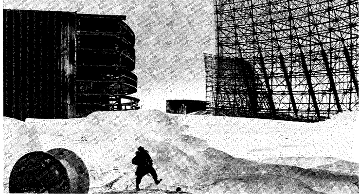
Fig. 3—Just one of many construction problems.
