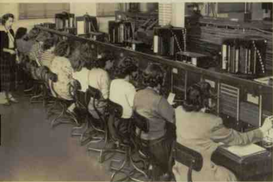
Fig. 1—Radio-telephone switchboard. Hub of network serving 2400 coastal vessels, 320 land stations and 60 mobile subscribers. Handles 25,000 calls per month.
