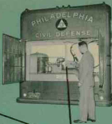
Fig. 6—D. Upton examines 10-kw Onan emergency power generator.
