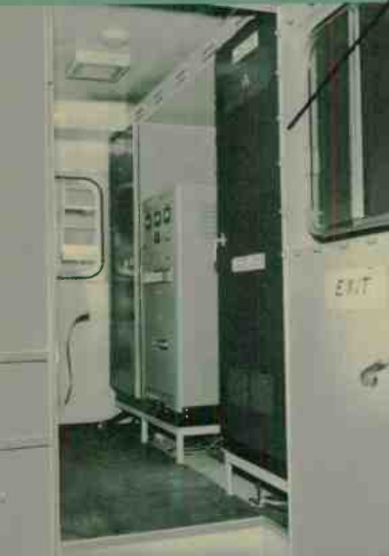
Fig. 4—Transmitter room houses police, C.A.P., and fire radio.
