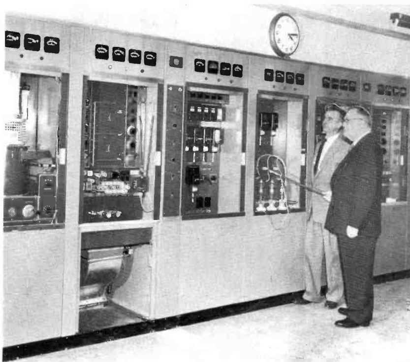
FIG. 5. The 50-kw RCA transmitter in the WGN-TV transmitter room on the 40th floor of The Prudential Building, Chicago. W. R. Crama (left), WGN-TV transmitter supervisor, looks over installation with Carl J. Meyers, engineering manager for WGN, Inc.
