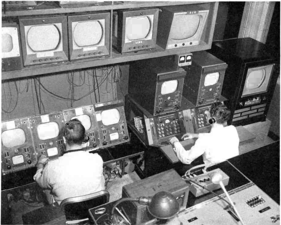
FIG. 18. Lower level of studio control room, showing video control equipment. At left, monochrome; at right, color.
