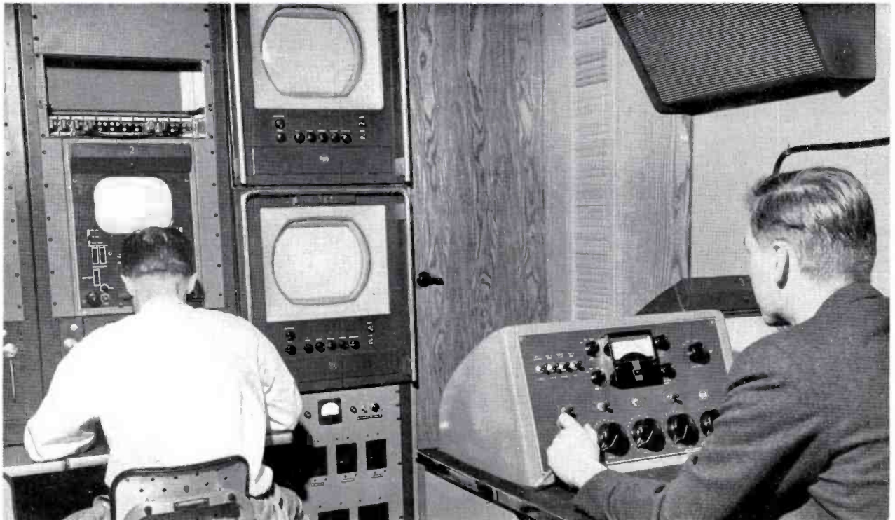
FIG. 13. Inside the color mobile unit at South Broad where the major part of the Mummers' Day Parade originated. From left to right are the TM-6C master monitors, the two TM-10B color picture monitors, a BC-4 audio console and another TM-6C master monitor.
