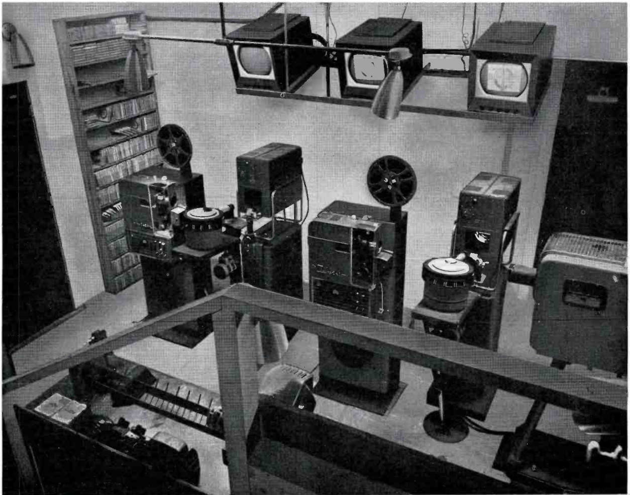
FIG. 17. View of WSUN-TV film room. Two RCA TP-6A Professional Film Projectors are shown, each with an individual TK-20D Film Camera. Multiplexed with the film projectors are two automatic slide projectors, and to the right, a Gray Tel-Op. Above are three RCA Utility Monitors.
