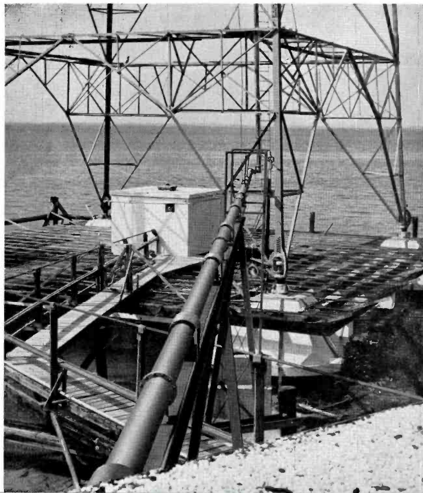
FIG. 7. View showing 6 1/8 " transmission line leaving transmitter building and method of supporting horizontal run to the tower.
