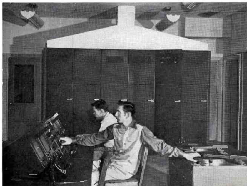
FIG. 10. Side view of the video operator's position. Video test and power supply racks are visible.
