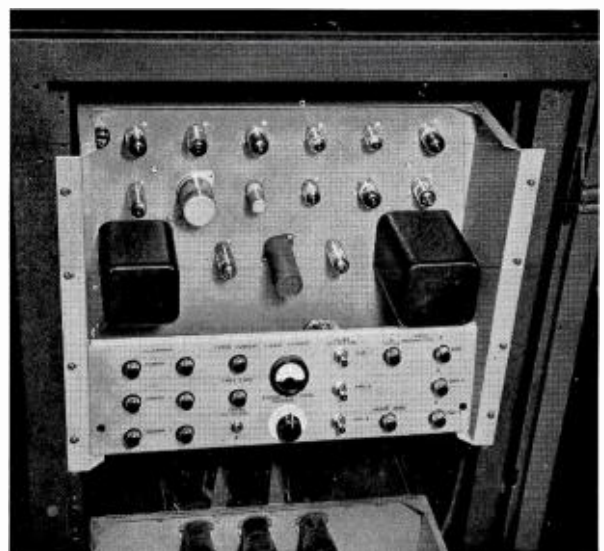
FIG. 10. Auxiliary Control Unit.
