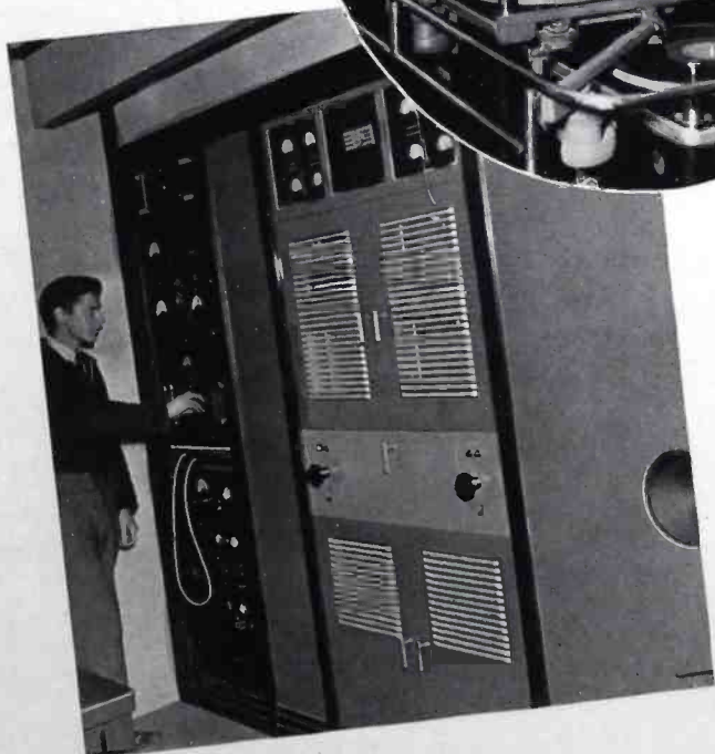
The RCA 250D transmitter in operation at WDAN.
