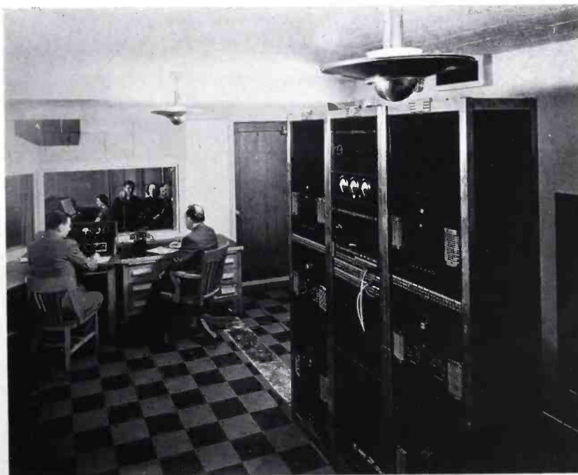
Looking out of the RCA Equipped Control Room into Studio A. An institute student program is in progress.
