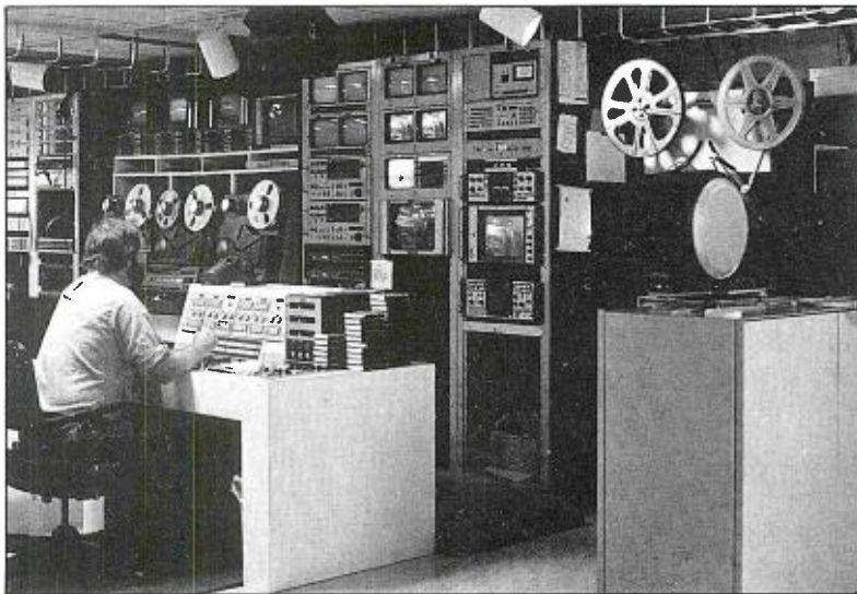
Master Control and technical area
