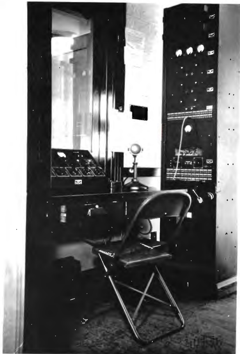
Corner of the control room at KSD showing RCA equipment in position
