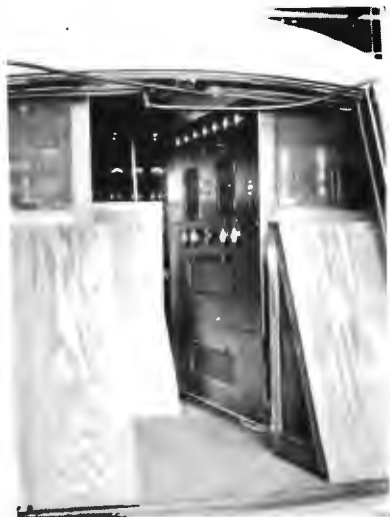
As a part of the equipment appears in the rear of the unit.
