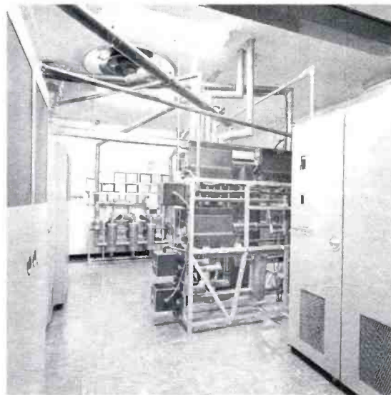
New TV-12 transmitting system includes OPTO-Switcher for optimum VSWR. Entire system was optimized on site before going on-air.
