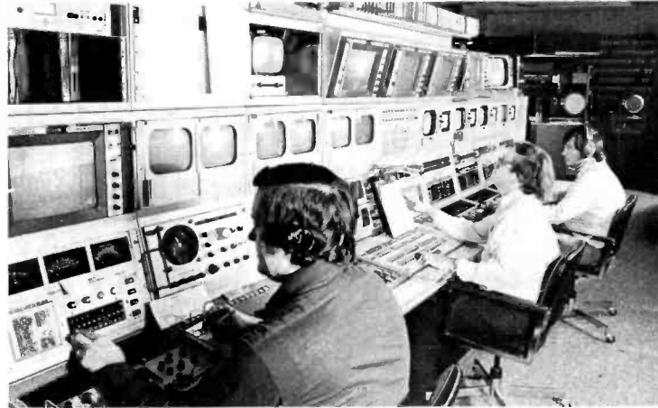
Compact control console line-up Includes transmitter remote controls; switching and machine controls; and TK-44 CCU's.
