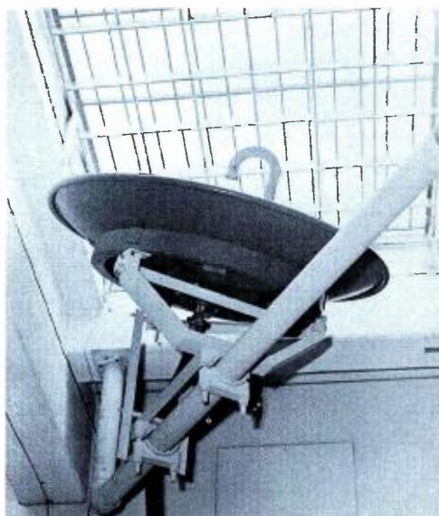
(Inset) Microwave dish for KSD-TV STL is mounted inside the transmitter building, protected by a heavy duty plastic covering and 8-inch steel mesh.
