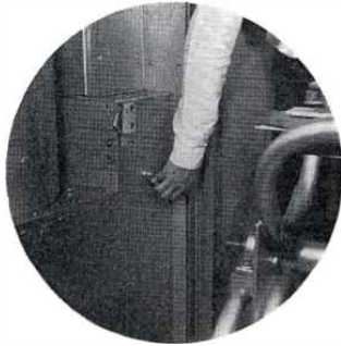
FIG. 5. Open collector drain valve.
