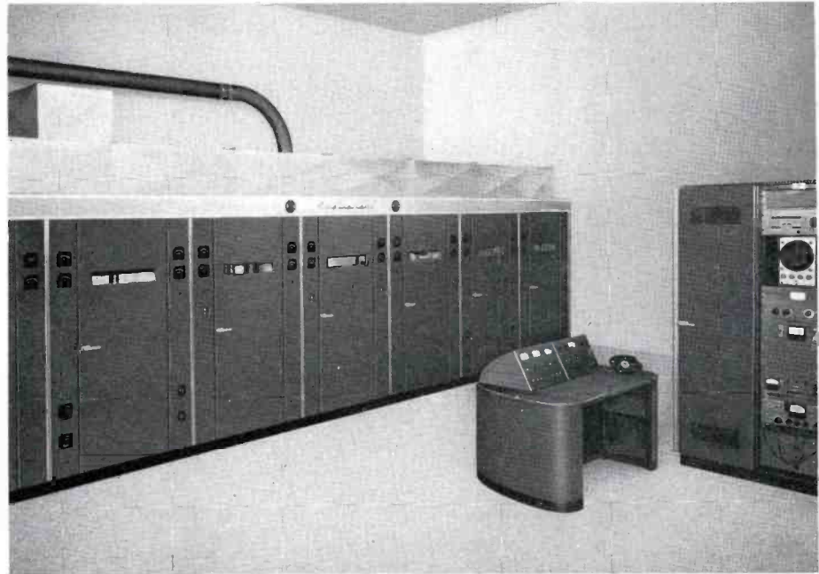
FIG. 2. Recent high power projects included building of this 250-kw Ampliphase transmitter now in operation at XERF in Mexico. This unit uses the basic Ampliphase concept at the higher power level.
