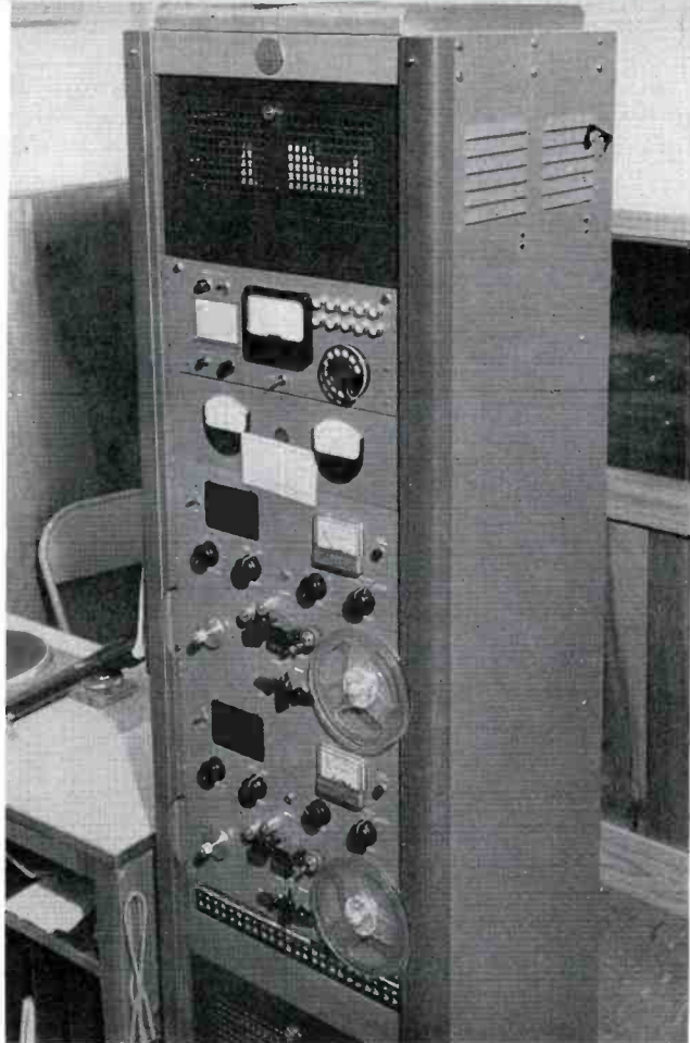
FIG. 2. Directly behind the control position is this rack of equipment. Transmitter remote control equipment, tape recorders, and the usual audio equipment for the entire station are conveniently located in the single rack.
