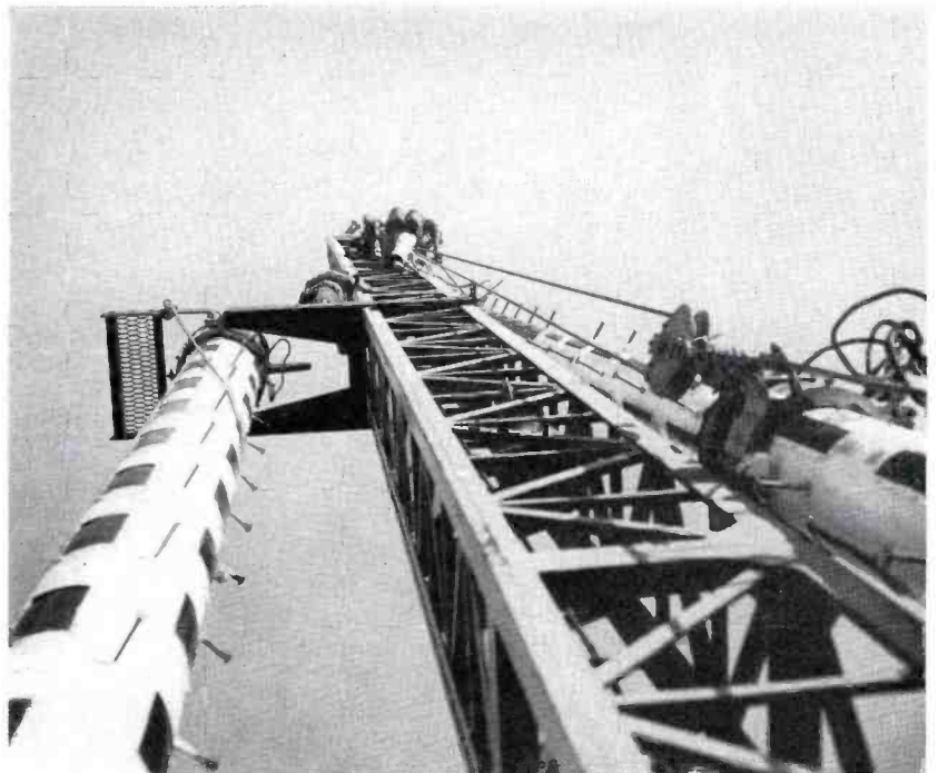
FIG. 7. Ease of installation is shown here, as the top section of the WIS TW antenna goes up the side of the tower. Special lifting clamps are supplied for raising the sections to the top of the tower.
