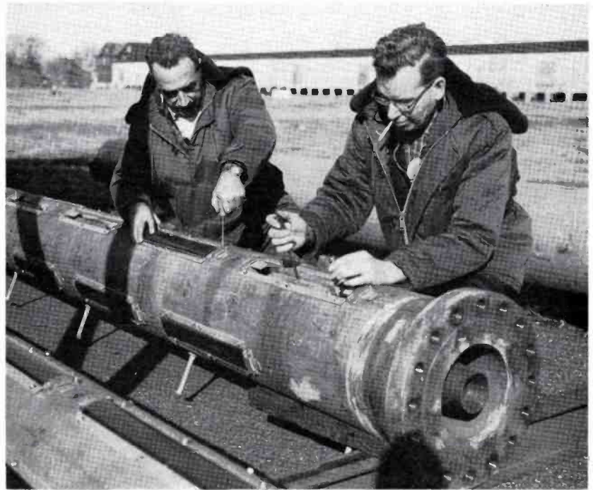
FIG. 2. Tuning plates and slot covers are attached before the TW antenna undergoes line tuning. Note the hollow inner conductor which is used to run lightning protector and beacon cables to tower base.
