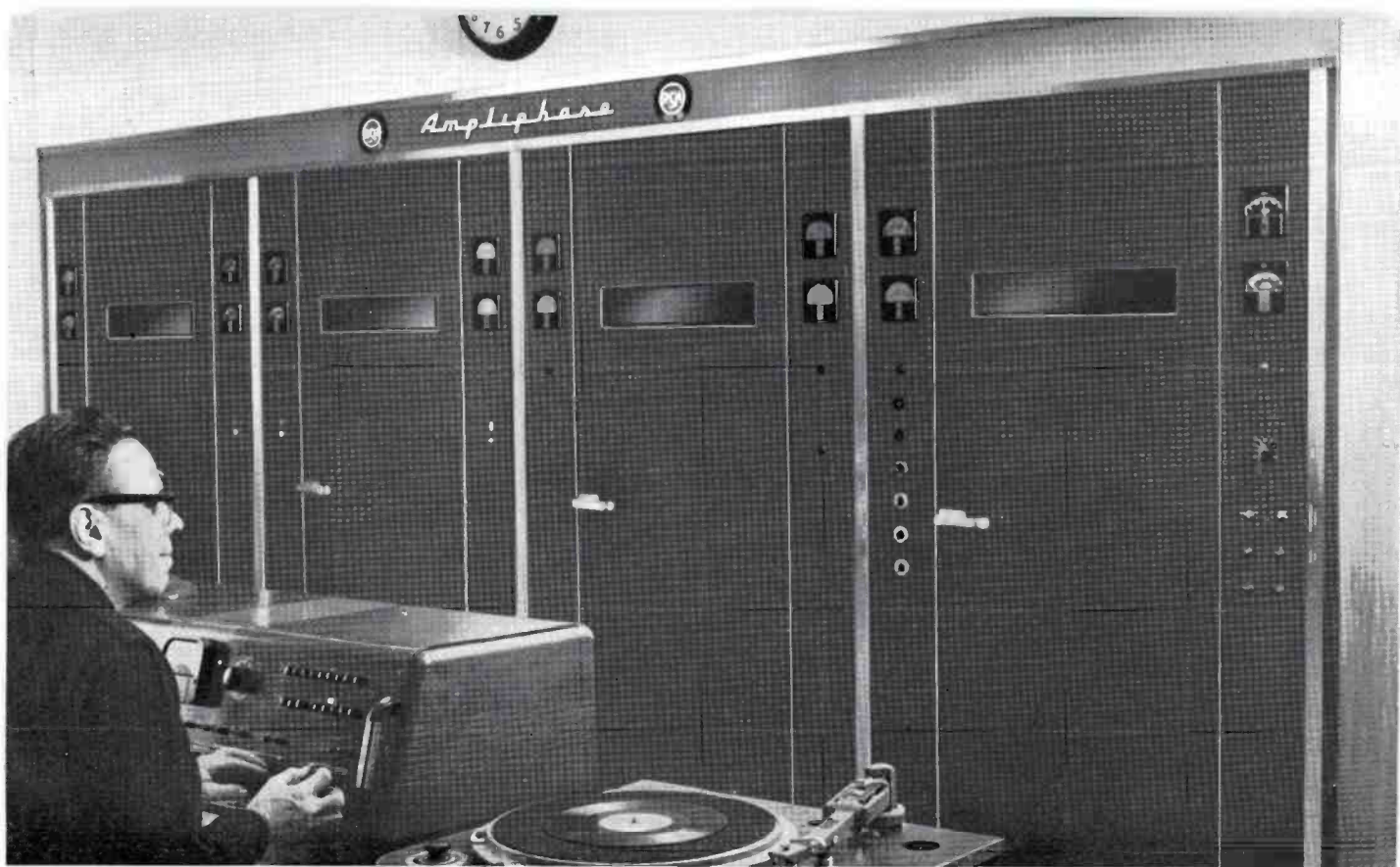
RCA Type BTA-50G transmitter at the WINS transmitter building in Lyndhurst, New Jersey, showing Al Jorgenson at Consolette.
