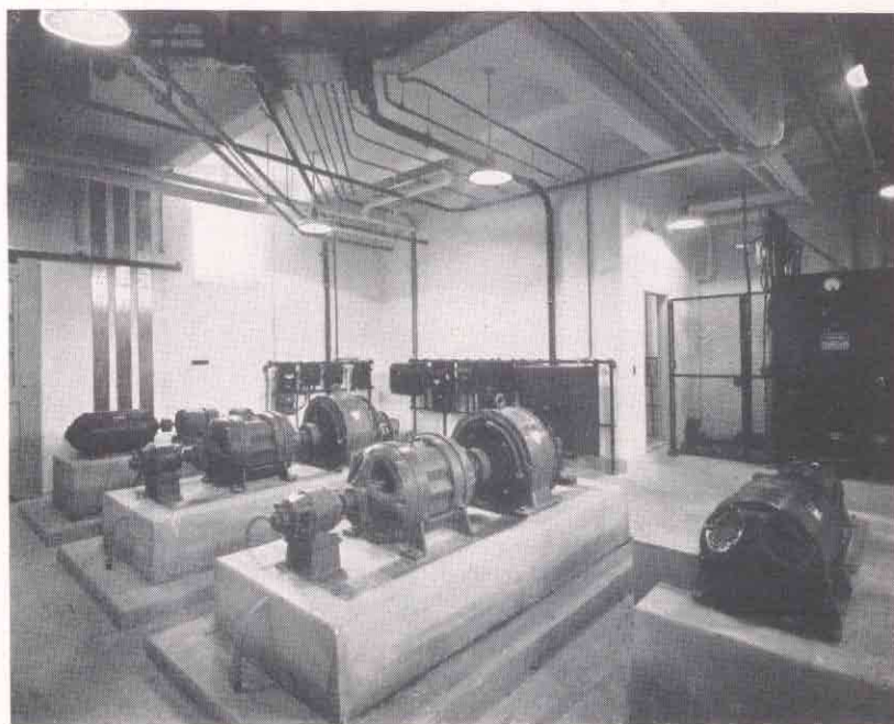
POWER ROOM WBT
