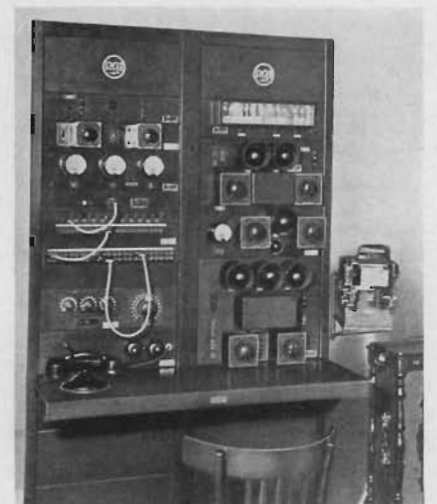
Fig. 7 CONTROL ROOM OF STATION IRO.—AN RCA VICTOR 50-B TRANSMITTER AT ROME, ITALY
