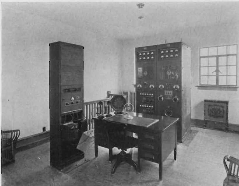
INTERIOR OF THE CONTROL ROOM
