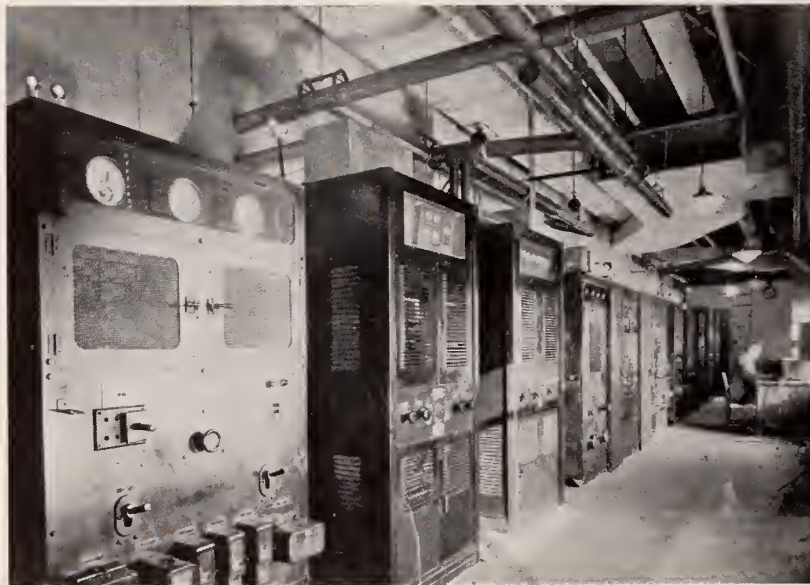
Empire State Transmitters—85th Floor
